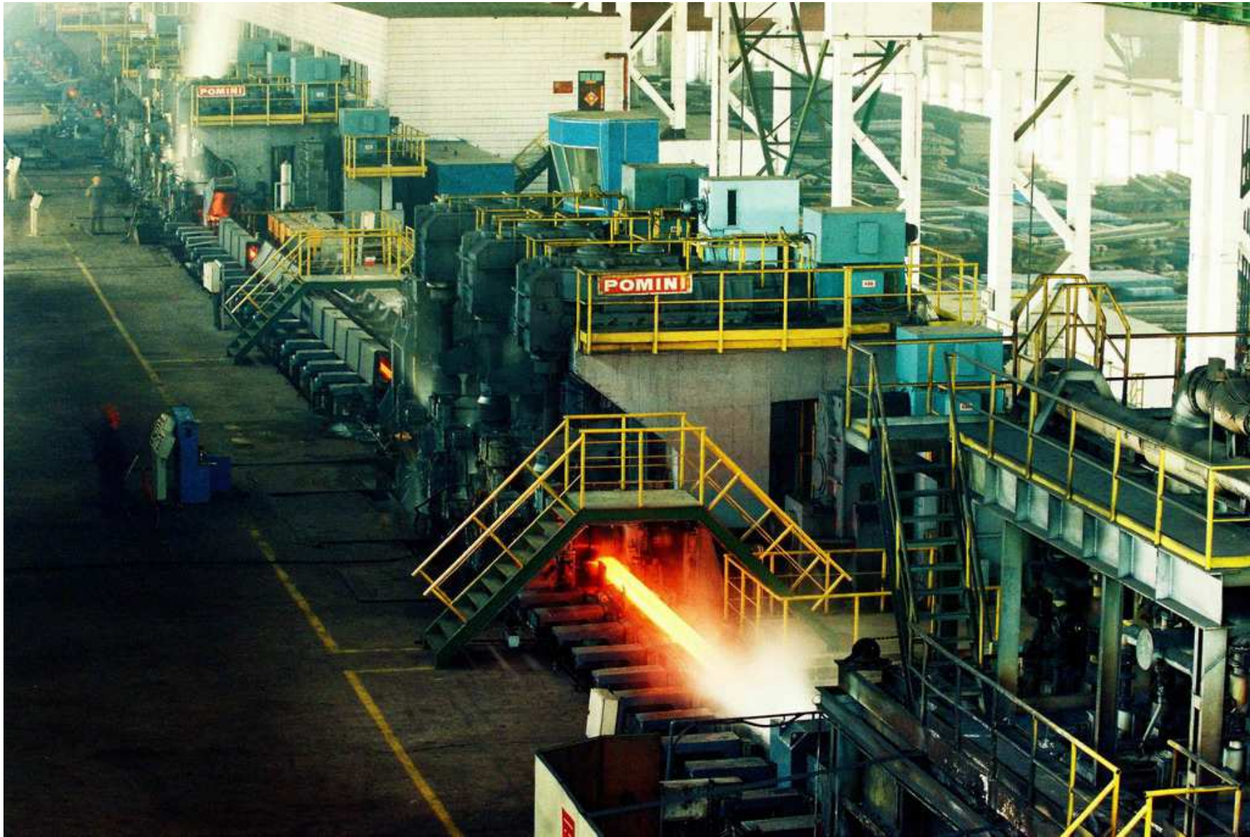
Bar rolling mill : H-V×24 stand/POMINI (Fushun)
